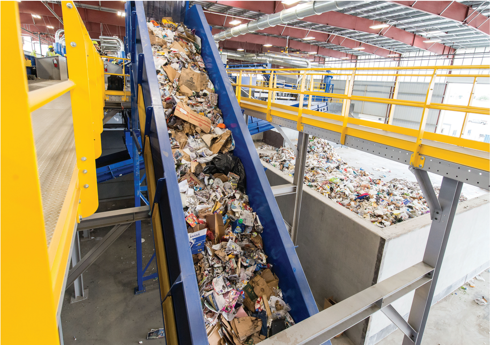
An impressive comeback: Anaheim Recycling Center is now one of Republic Services’ largest and most advanced facilities.
